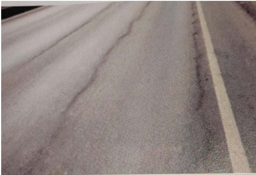
Photo 6.4.4 shoving of Bituminous Surface
