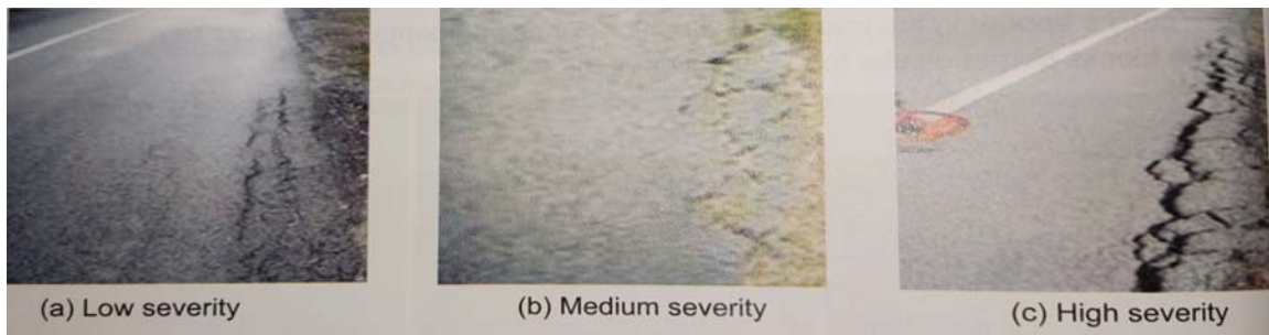
Photo 6.3.6 Severity level of Transverse Cracks
