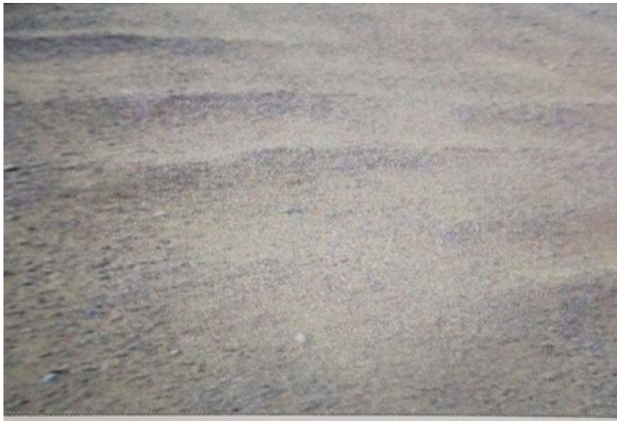
Photo 6.4.3 Corrugation of Bituminous Surface
