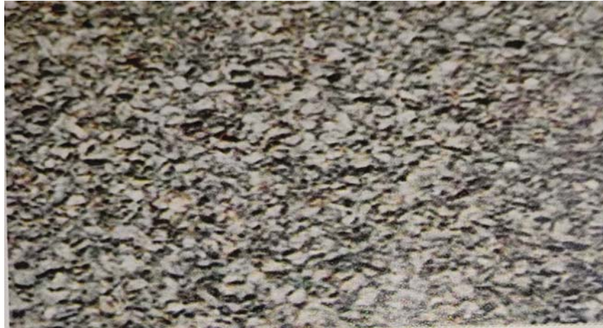
Photo 6.5.1 Stripping of Bituminous Surface
