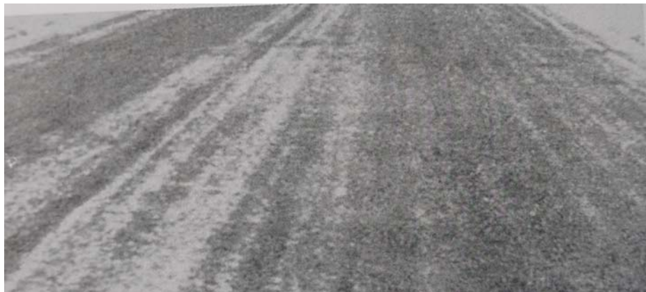
Photo 6.2.3 Streaking of Bituminous Pavement
