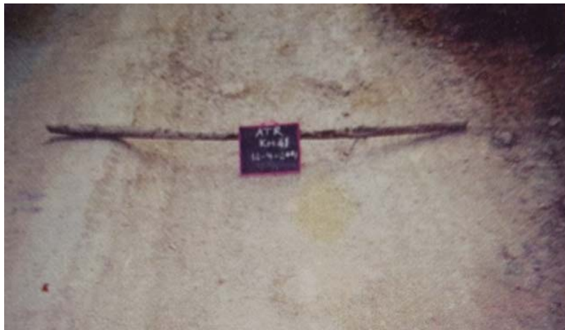
Photo 6.4.6 Settlement in Bituminous Surfacing
