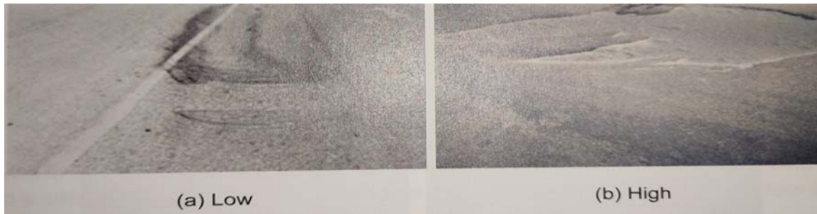
Photo 6.4.1 Slippage of the Bituminous Wearing Coat
