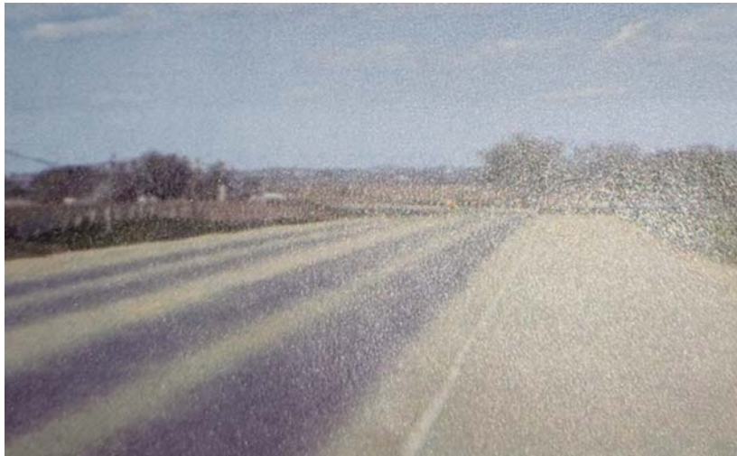
Photo 6.4.7 Upheaval in Bituminous Surfacing
