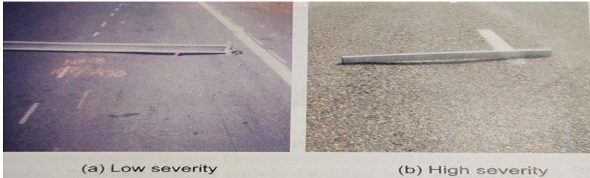
Photo 6.4.2 Rutting in Bituminous Surface
